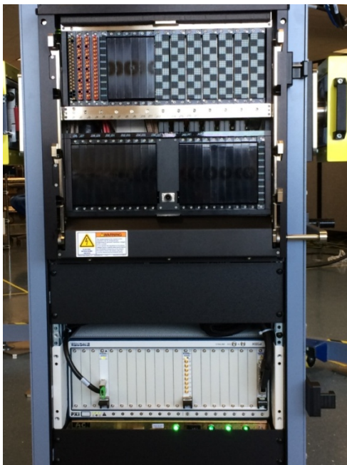
Figure 12: No Funnels for the PXI Instrumentation. The cables run directly to the existing user interface.
